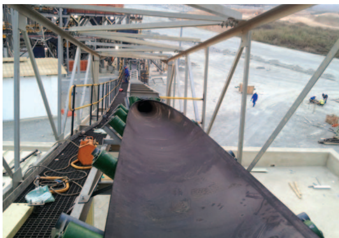
Pipe conveyor at Koidu Mine in Sierra Leone.
