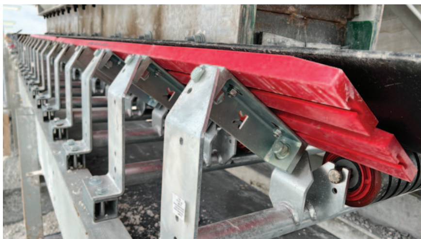
Conveyor belt support & conveyor skirting.
