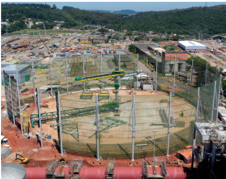
A WeatherSolve Structures cathedral style wind fence with conveyor access points for a wood chip stockpile in South America.
