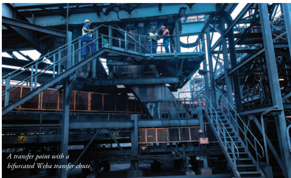
An incoming belt feeding a head chute at a coal mine.
