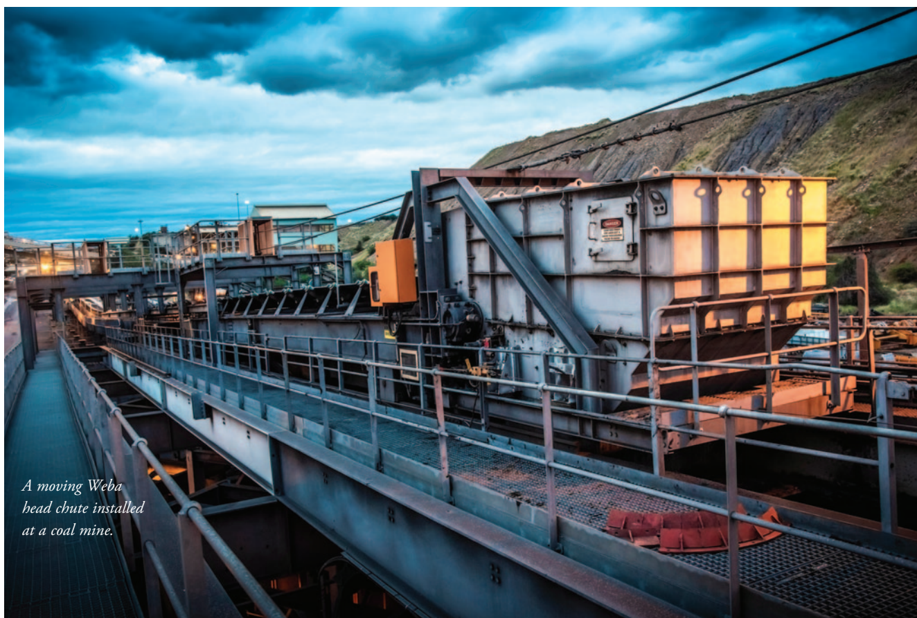
A transfer point with a bifurcated Weba transfer chute.
