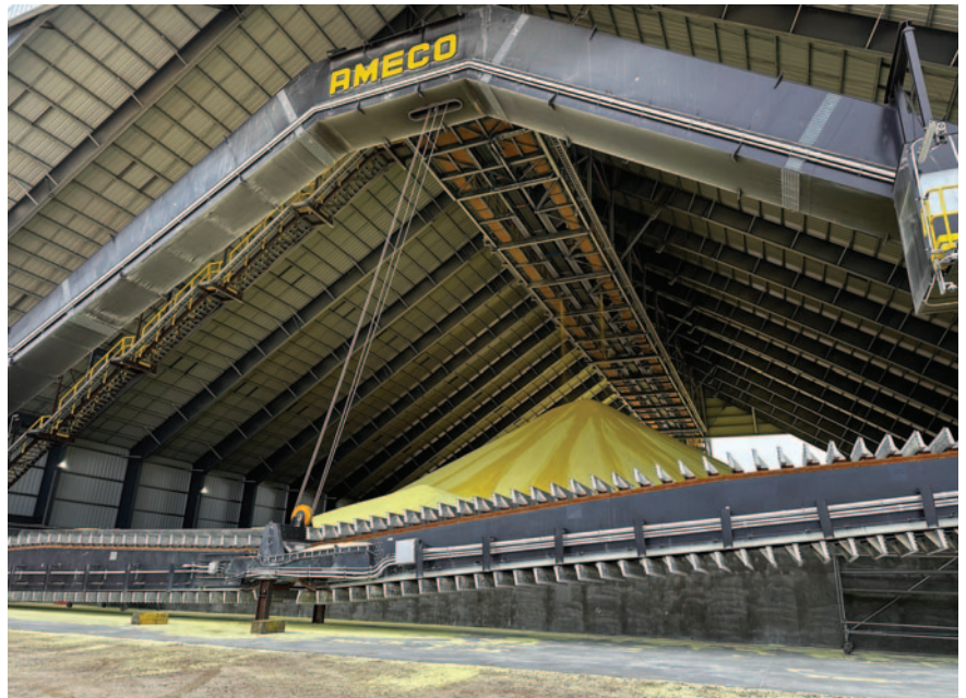
Fire & Ice: where Arctic temperatures meet flammable product, safety handled by one of AMECO's largest reclaimers.
