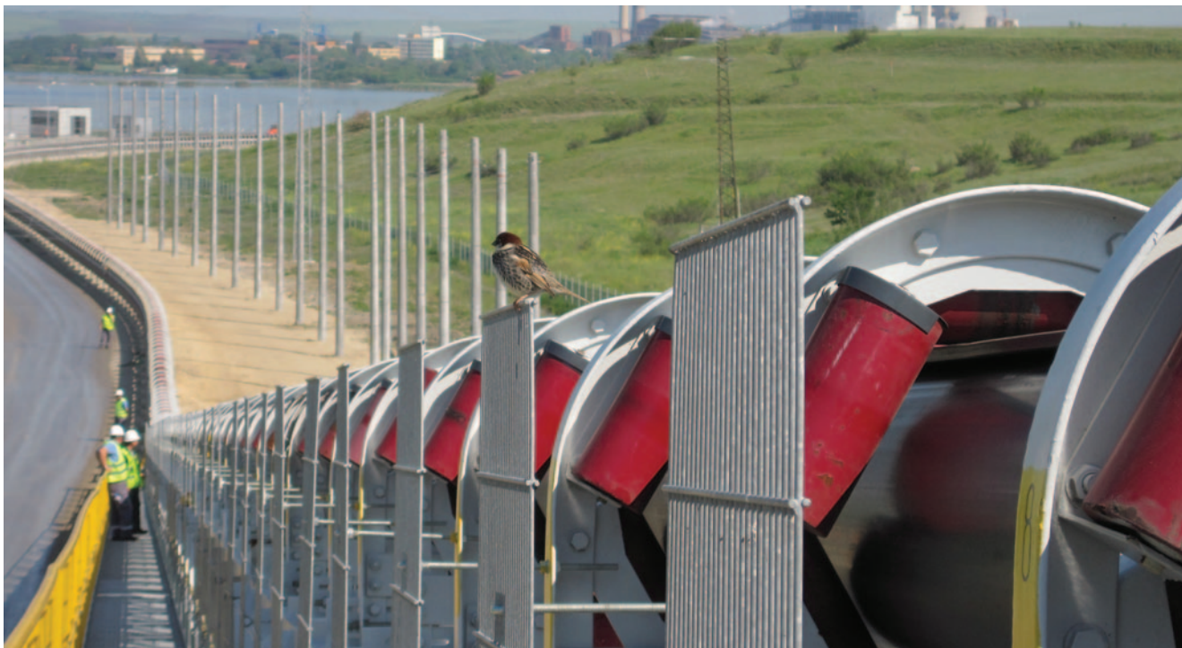
TAKRAF Tube Conveyor with a capacity of 1,400tph in Bulgaria.
